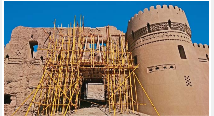
The 2003 earthquake destroyed lots of buildings in Arg-e Bam but part of them have been rebuilt and some parts are still under construction.
